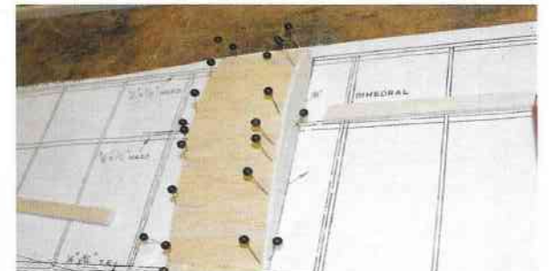
Construction of the wing in one piece, starting with the centre section...
